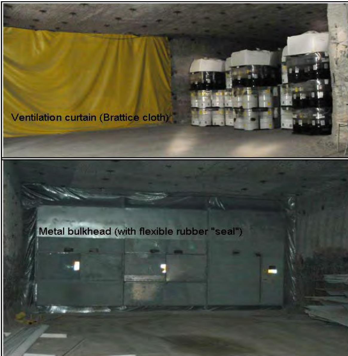
Fig. 2 Photos of a typical ventilation barrier called a brattice curtain (top) separating each disposal room, and of a typical metal bulkhead (bottom) “sealing” the inlet and outlet drifts of each disposal panel from ventilation air in the rest of the mine.
